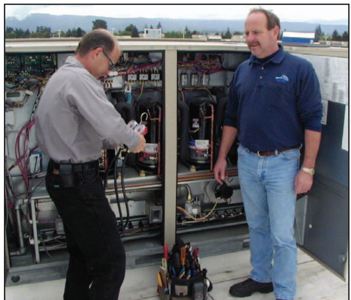
Top: Ikea is known for being socially responsible, so for its latest three stores in California, the company decided it wanted to install rooftop units containing R-410A. Above: Cal-Air employees Mike Camper, area foreman, and Guy Booten, field operations manager, perform the preventive maintenance on the rooftop units.
