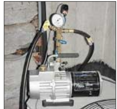
A vacuum pump is connected to an air-conditioning system during refrigerant evacuation. Both a mechanical-dial and thermocouple-style gauge are used together to optimize measurement accuracy.
